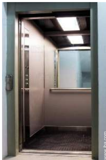
Equipment at the guest's disposal
